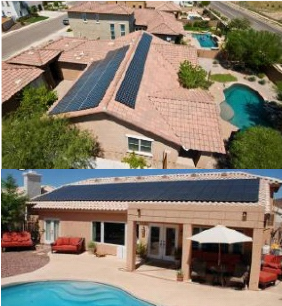
The solar panels shown above are low profile and are parallel with the plane of the pitched roof.
